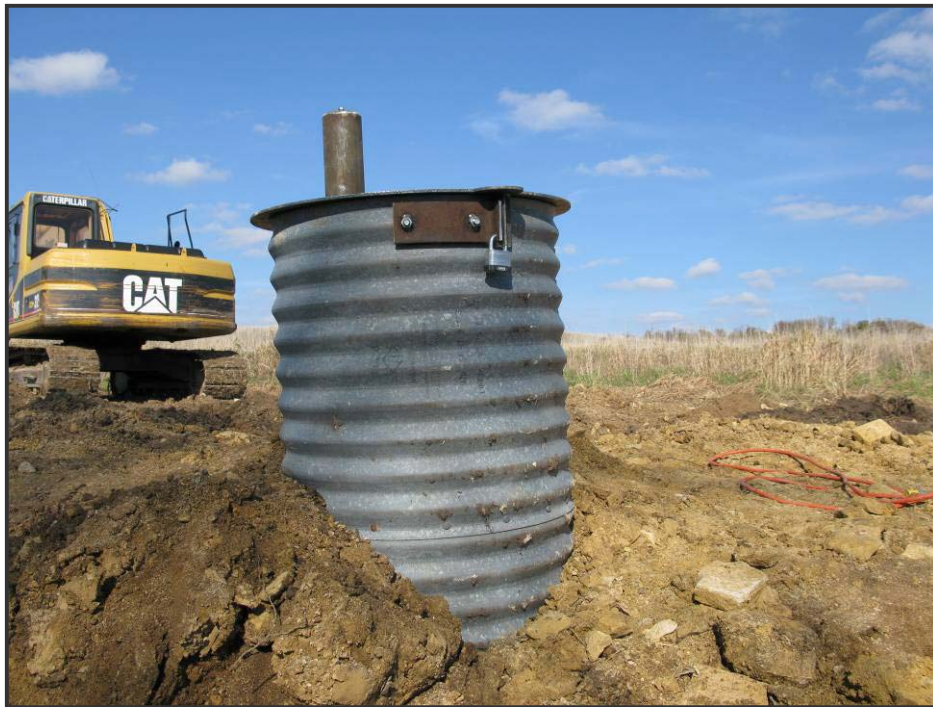
The new entrance will be located about 350' away. Once the new entrance is completed this temporary entrance will be removed. The site will be graded and replanted with native grasses.
