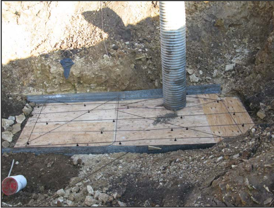
Sheets of tin were placed along the perimeter to form a tight seal. A temporary culvert access to the cave was installed.
