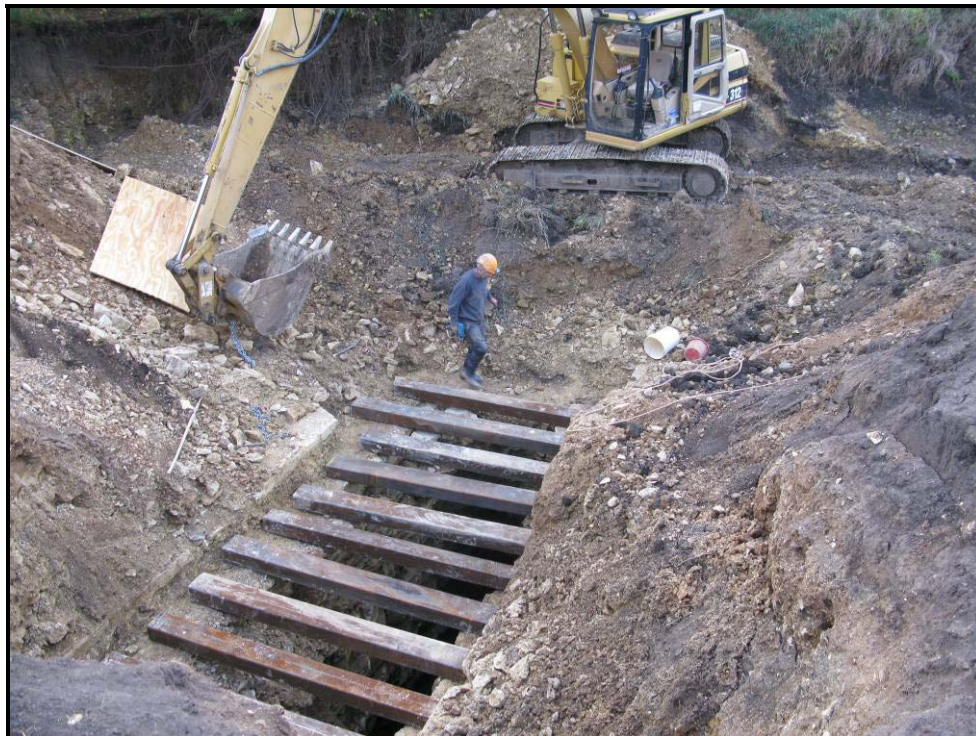
After the bedrock was exposed, structural steel tubing was placed over the open hole. Then thick plywood was placed over the beams and rebar was installed.
