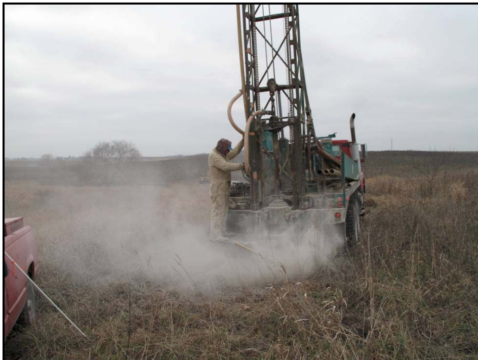
A small test hole has verified the accuracy of the new shaft entrance. Next up: A large industrial drill rig and a host of support equipment will now arrive to create the actual entrance.
